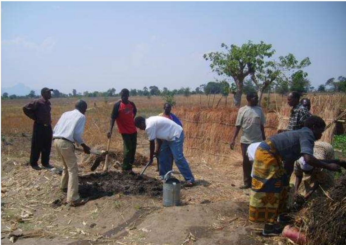
Community members with LCD staff preparing mud to seal the compost manure heap
